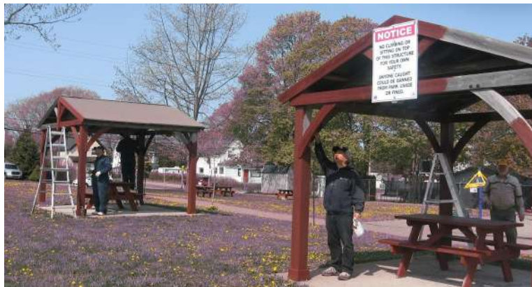
Several members of the Amherst Lions Club gathered at the Lions Park on a sunny day to stain 3 old Gazebos. The Gazebos are in much use by the community but were getting a bit shabby looking. Here the lions are hard at work and the results were a great improvement.
